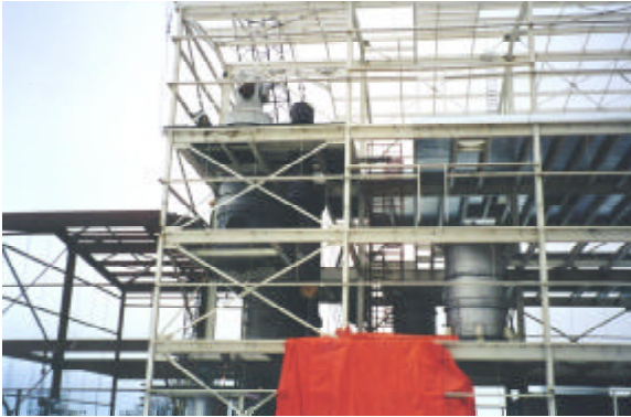
Refinery Bldg frame with Deodorization/Bleaching Vessels
